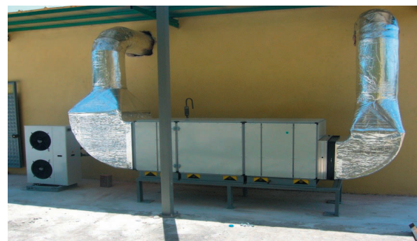
D) Air conditioning unit
