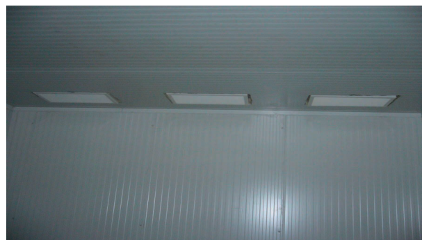
C) inside of the cold storage
